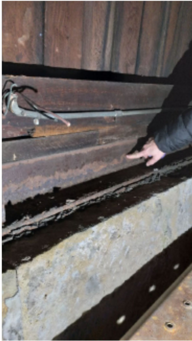
Figure 5. Interior of Dome showing line of rusted steel on L-angle base plate probably caused by water ingress.
