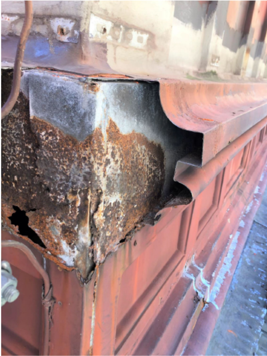
Figure 7. Dome Lantern, showing the deteriorated condition of the original galvanized steel sheet.
