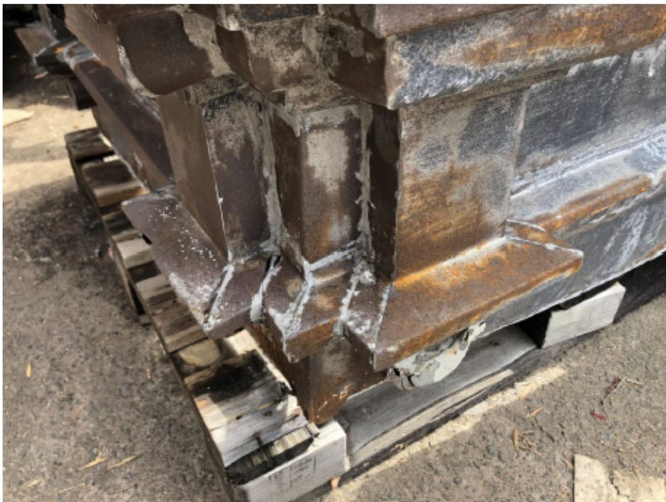
Figure 6. Dome cupola cladding showing the loss of galvanising and associated corrosion.
