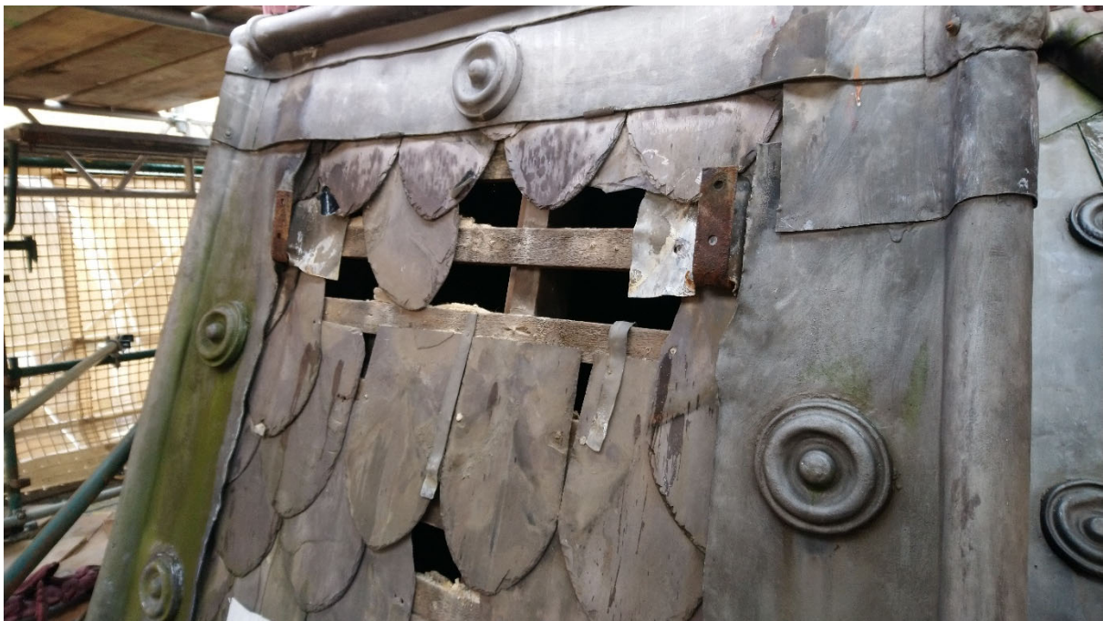
Figure 2. Deterioration to turret.
